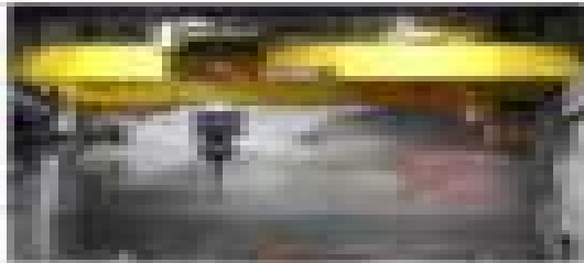
This class "B" generating station crane is rarely used.
